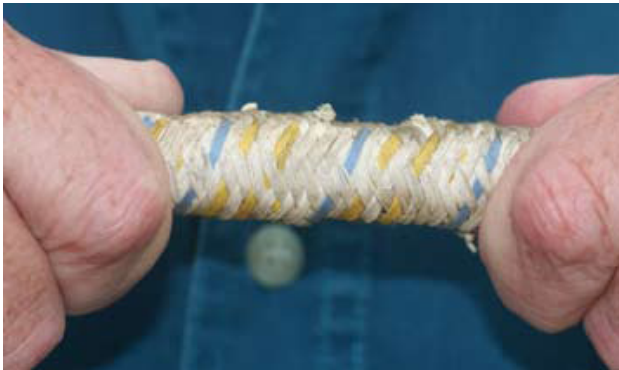
Most normal humans would not be able to pull on a 3/4-inch shock cord and be able to stretch it, but this cord had deteriorated to such an extent that it was possible for me to do so!
