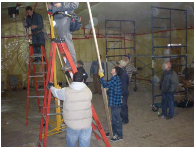
Arie Lazarus, Wilem Pokornik, Al Heim, Bob Hamel, Doug Render, Dale Chevalier, Vic Prefontaine, Gil Bourrier And Dani Pokornik installing drywall. December 2008 to March 2009
