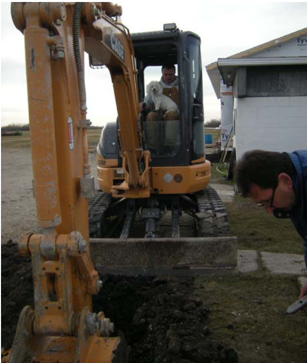
Perry Chromiec, Gil Frechette, Tom Stoyka, Gil Bourrier, Adrian Meilleur and Brian Kirk looking for hot wires feeding The maintenance building and some hangars. Dale Chevalier operating the excavator donated by Darco Ent. with his dog "Buddy"
